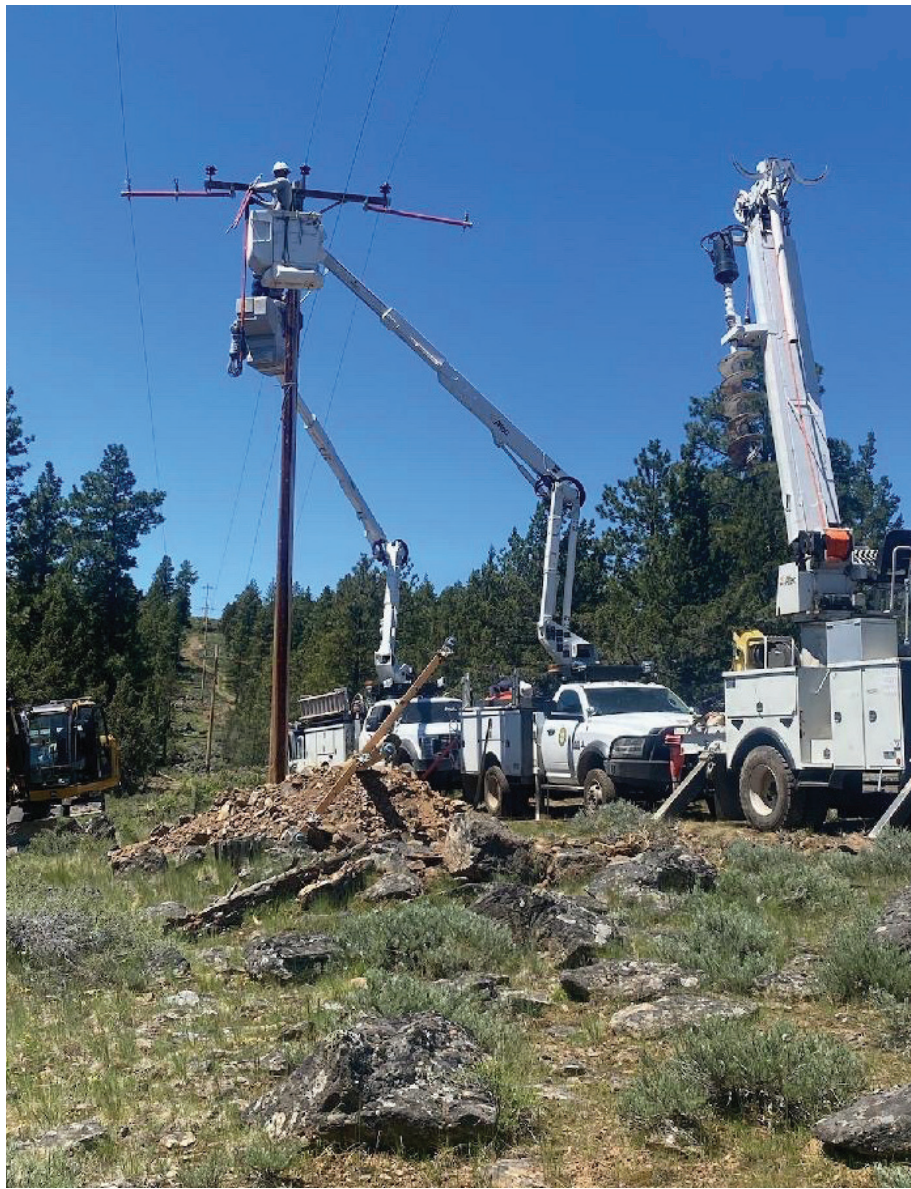
Oregon Trail Electric Cooperative crews perform maintenance and repairs in Baker County. PHOTO BY OTEC JOURNEYMAN LINEMAN CHRIS PEPPERS
